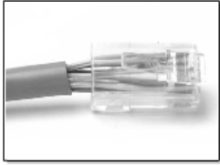
Bad Connector - Wires are untwisted for too great a length.
